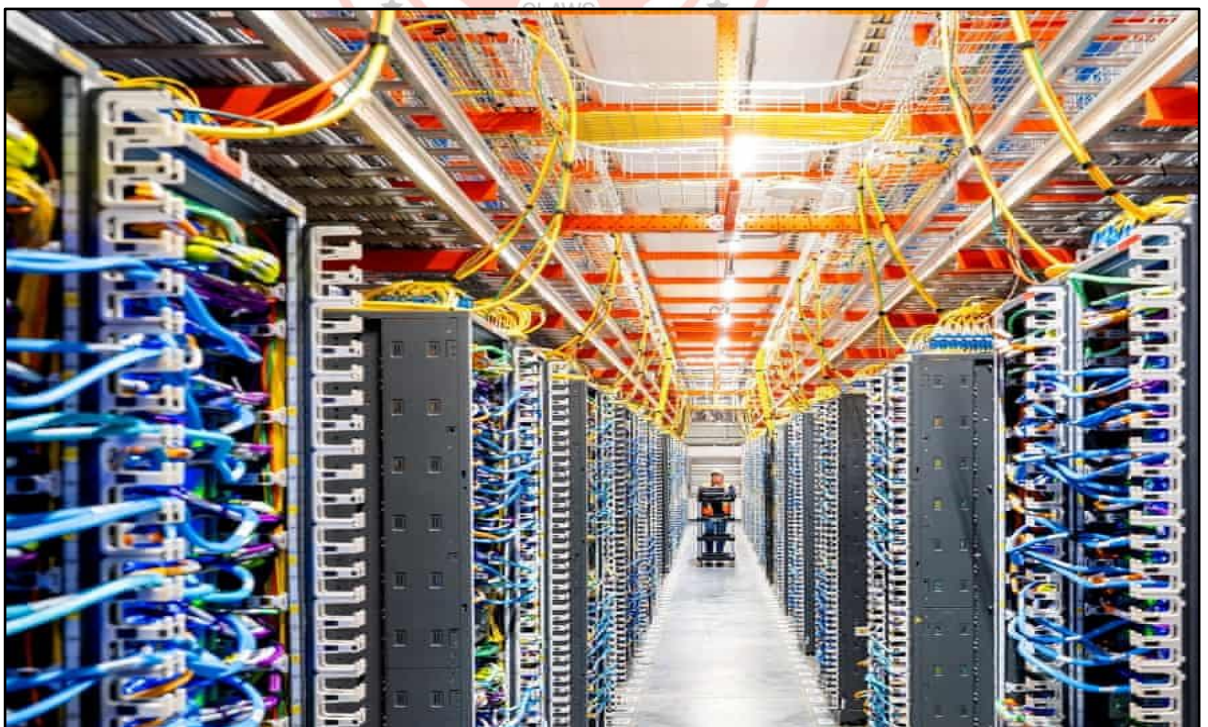
Figure 6: Representative Image of Data Centre
